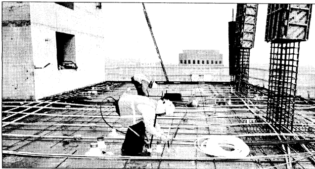
Day 3 – Subcontractors begin sleaving and roughing-in mechanical, electric and plumbing to the slab. Rebar work starts.
