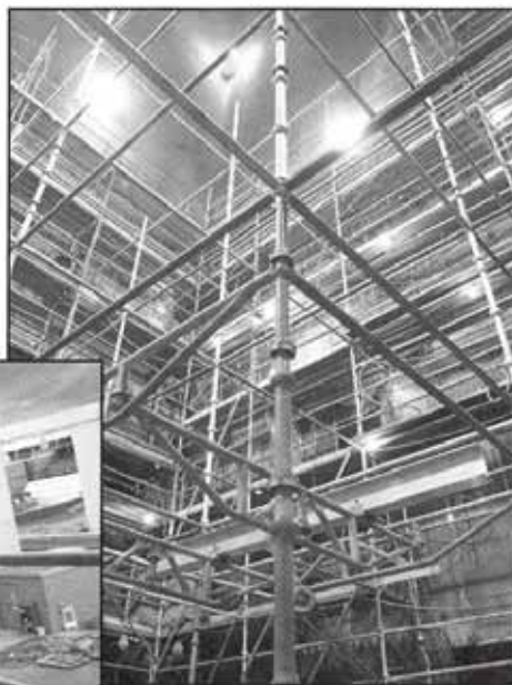
Brand's scaffold erected inside the boiler at Monroe Power Plant in Michigan.
