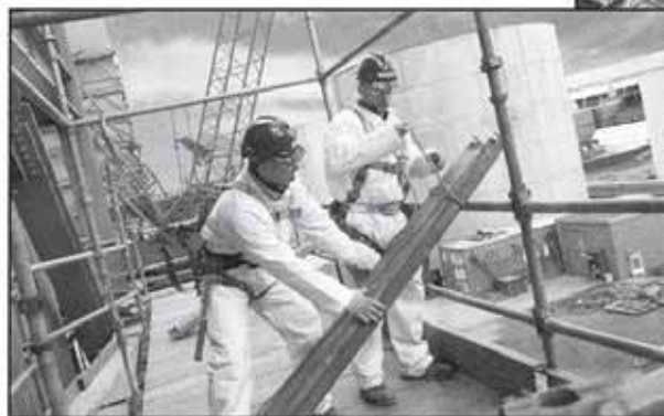
Brand's workers at a power plant.
